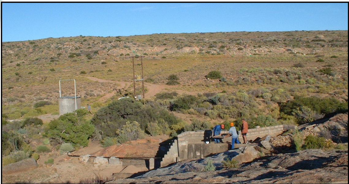
Figure 16: Sand filter with injection and abstraction borehole (pump house) in the background
